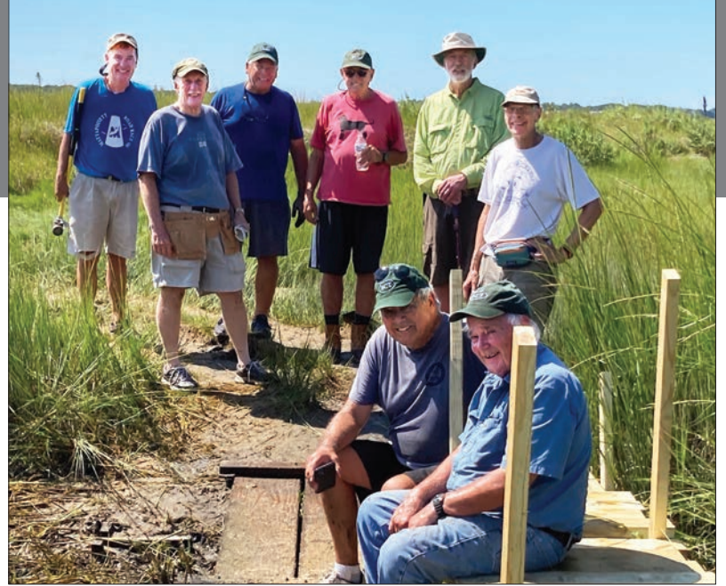
The Trailmeisters who came out on a "wicked hot" day, to build a bridge to Lawrence Island over the marsh. L to R: Matt Stone, Dick Murphy, Frank Guerra, George Gillis, Neil McPhee, Mike Lipchak, sitting are: Paul Rossi and Peter Fisher.
